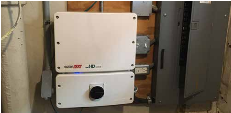
An Inverter (converting DC current to AC) is installed in the basement next to the electrical panel Photo by Jay Hoekstra
